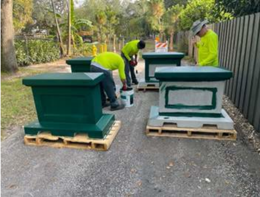
Preparing Concrete Barrier Wall for installation @ 69 th Ave (Ruffner/Roatta Dead End St)
