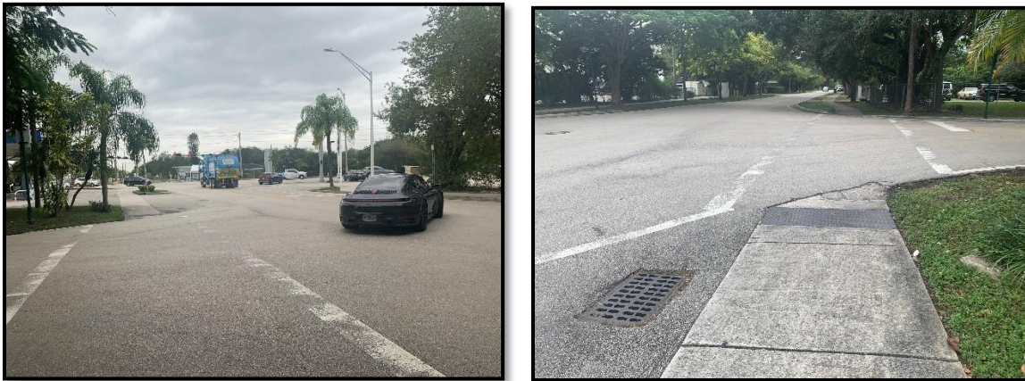
Figure 12 – Photos (crosswalk condition at SW 120th Street)
