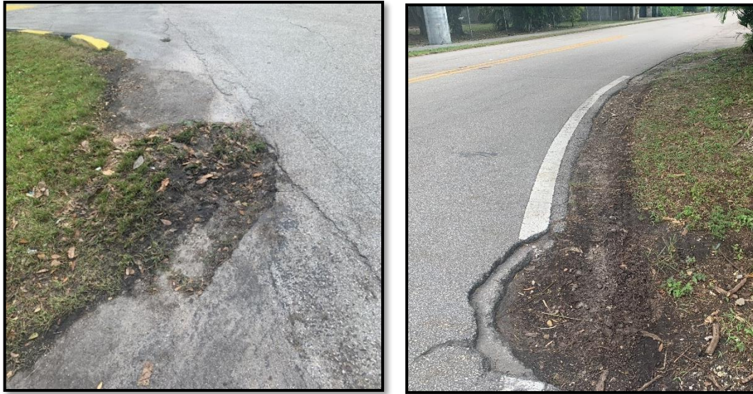
Figure 7 – Photos of worn roadway shoulder
