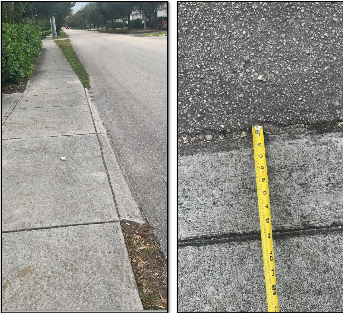
Figure 11 – Photos (left: sidewalk near travel lanes; right: sidewalk distance from travel lane)
