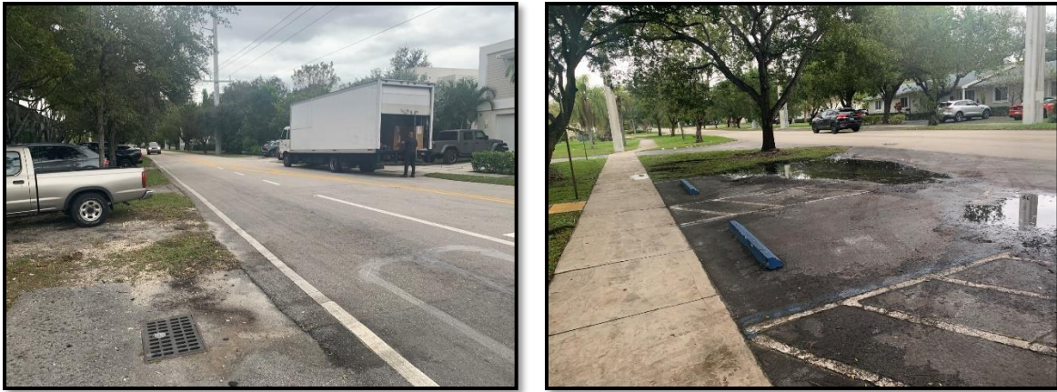
Figure 14 – Photos (left: inlet; right: ponding)
